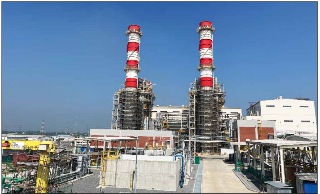
Meghnaghat 718 MW CCGP of Jera waiting for commercial operation since last April
