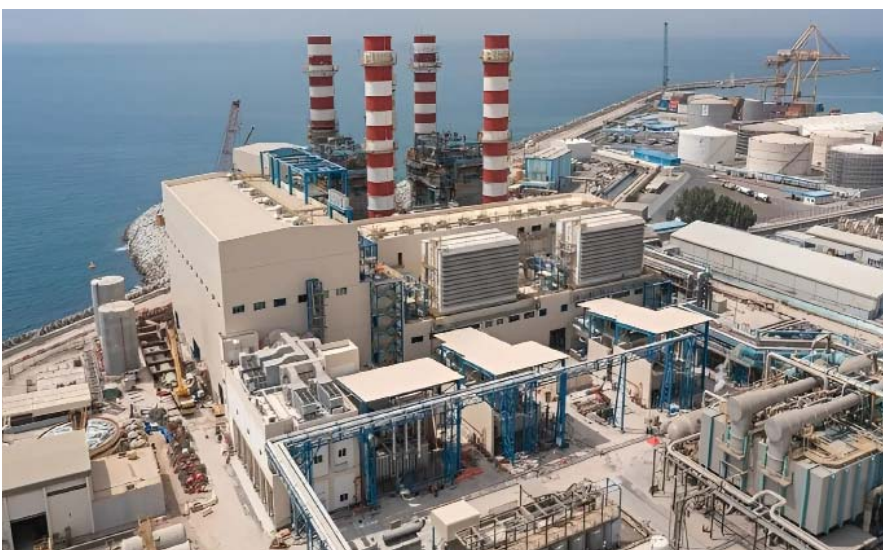
A view of Summit Meghnaghat II Power Plant
