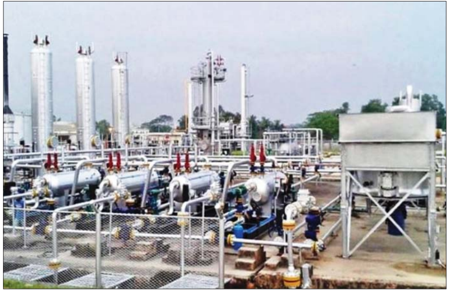
A process plant of Bangladesh Gas Field
