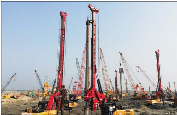
Piling activities Rampal 1320 MW Maitree super thermal power plant of BHEL by Dipon
