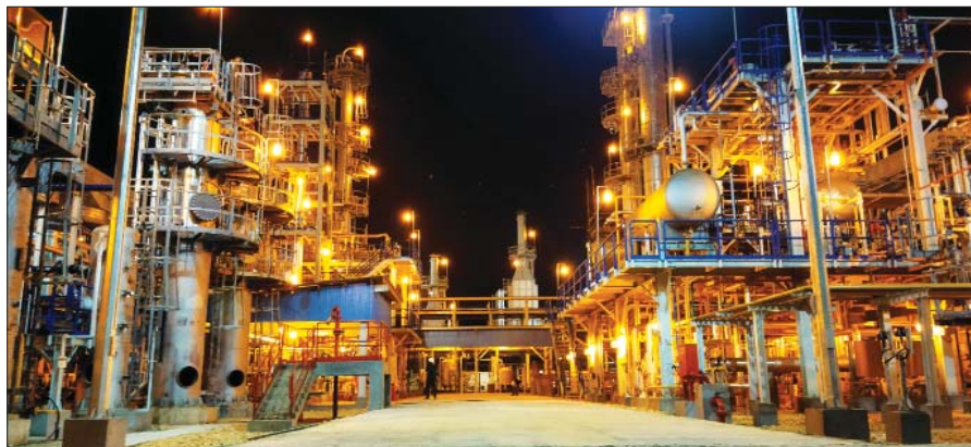
Catalytic reforming unit of SGFL, EPC done by Energypac
