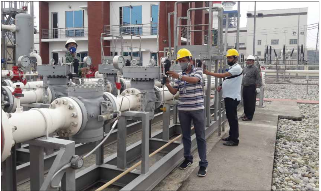
Gas pressure checking at a power plant of NWPGL
