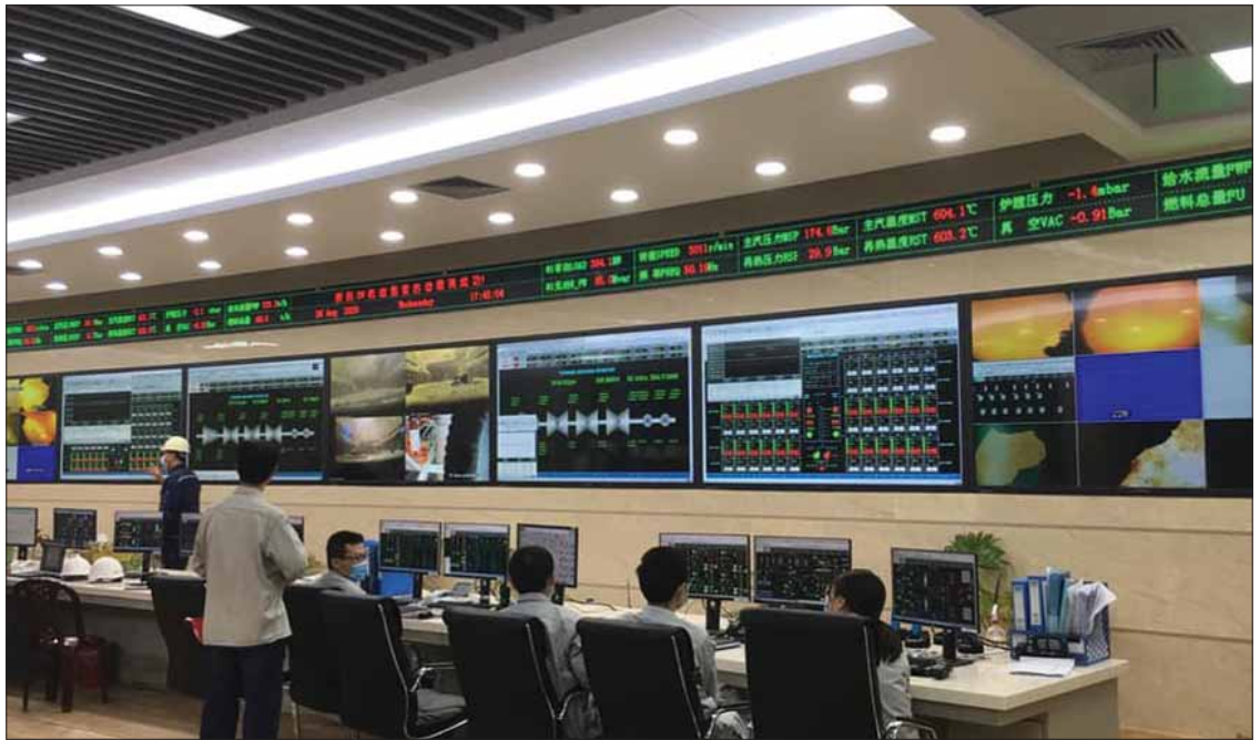
Payra power plant control room
